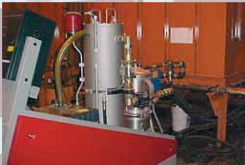
Dewatering Unit FAM and off-line filtration in hydraulic system using Quintolubric®.
