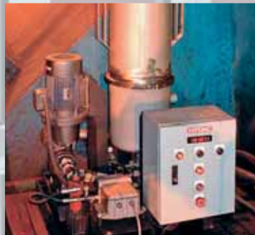
OLF Off-line Filtration with ContaminationSensor CS 2000.
